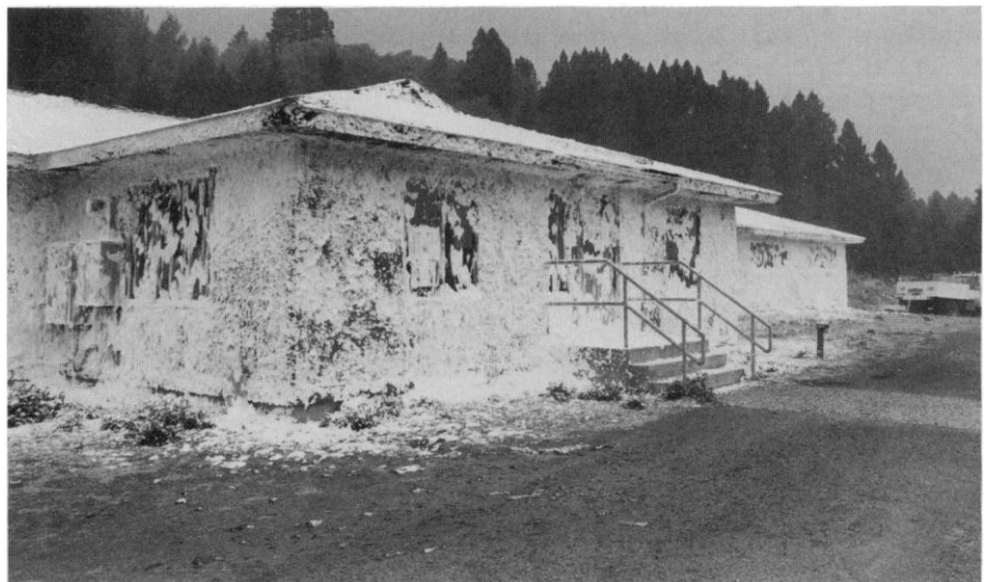
Figure 3. Fire-retardant foam was used on buildings, in this case a residence at Mammoth Hot Springs, 10 September 1988. Most buildings were adequately protected by such techniques. Photo: Jim Peaco, National Park Service.
